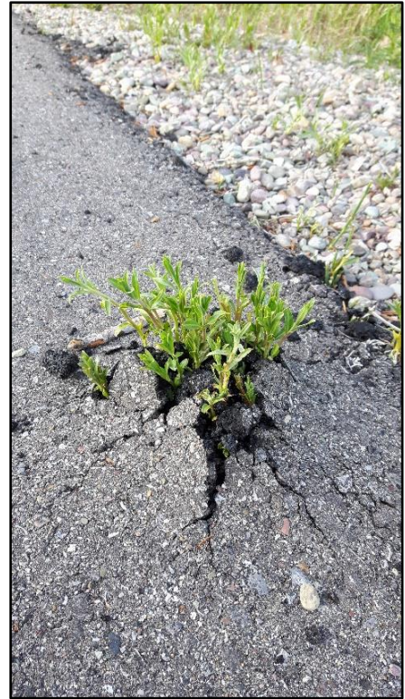
Ashphalt failure on inner loop of existing trail
