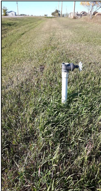
Picture 60 - Looking north at irrigation infrastructure within the east side of the 5 th Street W right-of-way
