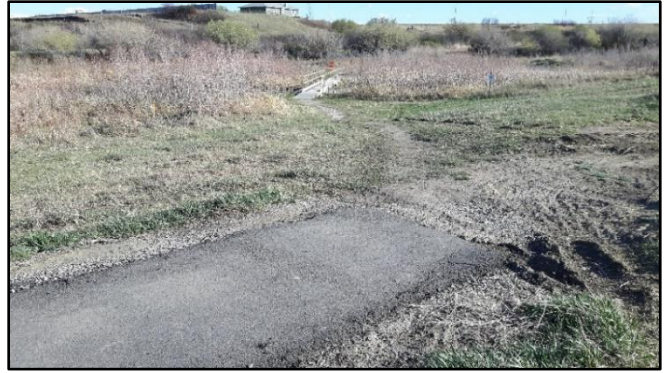
Looking south at surface transition in outer loop of existing trail (paved in August 2016)
